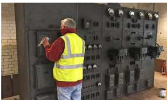
The Switch Gear being carefully conserved
